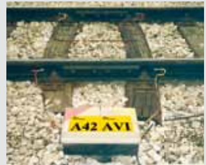
Rail circuit box
