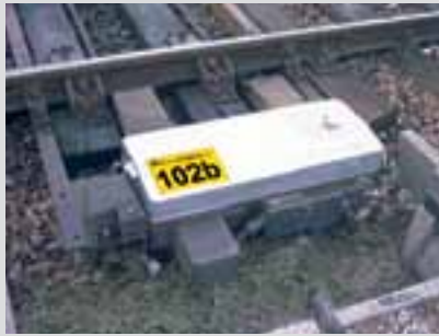
Switch shunting box
