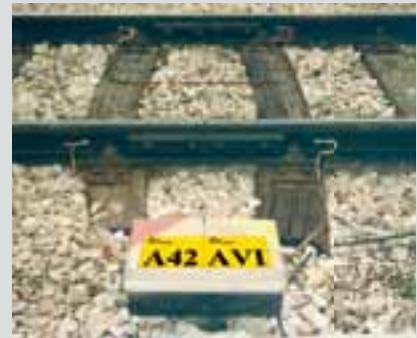
Rail circuit box
